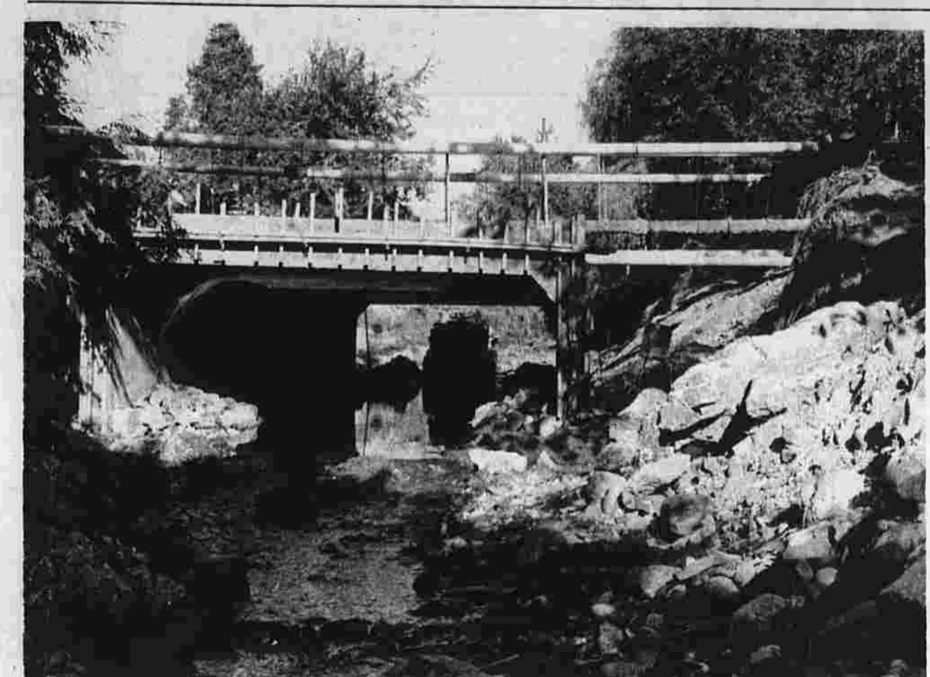
Bridge Construction on Schedule The new $60,000 bridge at the Bigelow Brook on Woodbridge St. is in shape. This week, work progressed to installation of pre-cast concrete units on footings poured last month. The box culvert structure is on schedule, Town Engineer Walter Senkow reports, and Wood-
